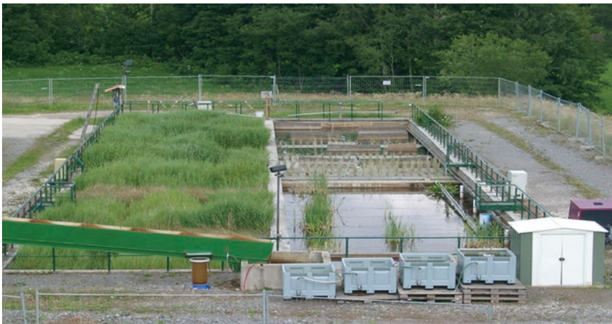
Fig. 9.17 Wisnut-designed mine water treatment system with rooted plants receiving water from the right side for treatment. On the right side, in the open water, Boojum recommended installing curtains for biofilm formation and floating cattail islands to address fine iron particles. In the foreground some cattail islands grew well, but others were plagued leaf lice. The light blue buckets were installed to provide a flow-through system for Chara . Growth data were used to derive design criteria for scale-up
